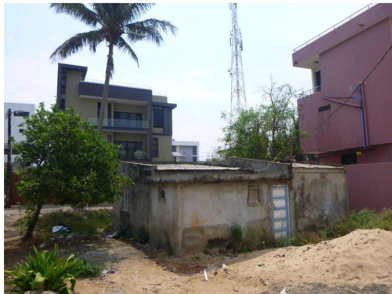
Figure 7. Subsidence of older houses in Triunfo (Photo by authors).
