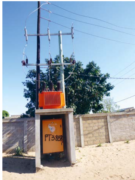
b) Transformer station
