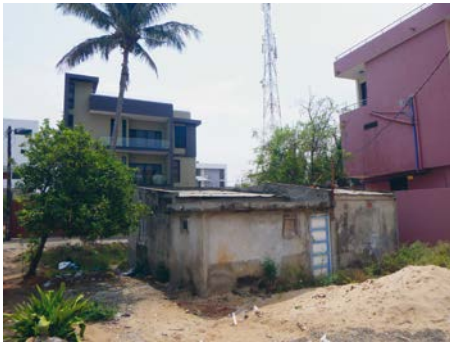
a) Subsidence of older houses
