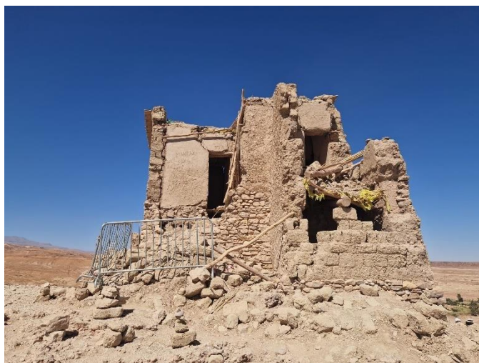
Figure 45: Collective granary in Aït Benhaddou, heavily damaged by the 2023 earthquake
