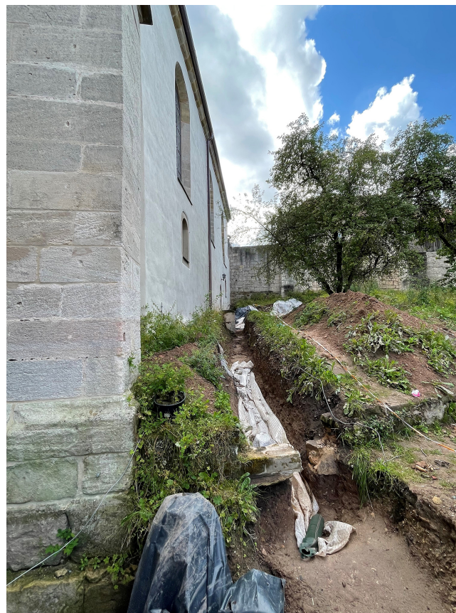
Figure 2. The excavation site at the northern side of Saint James Church, where the tin buttons were found.
